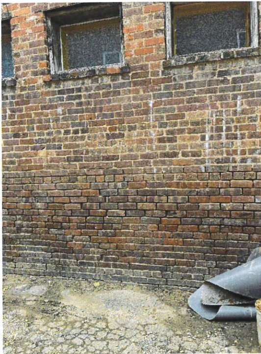
Mortar stripped from the bricks of 24 Commerce St
